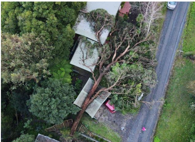
Wattle Avenue, from Susanne Richards' Facebook page. The tree demolished the carport, but missed the house.
